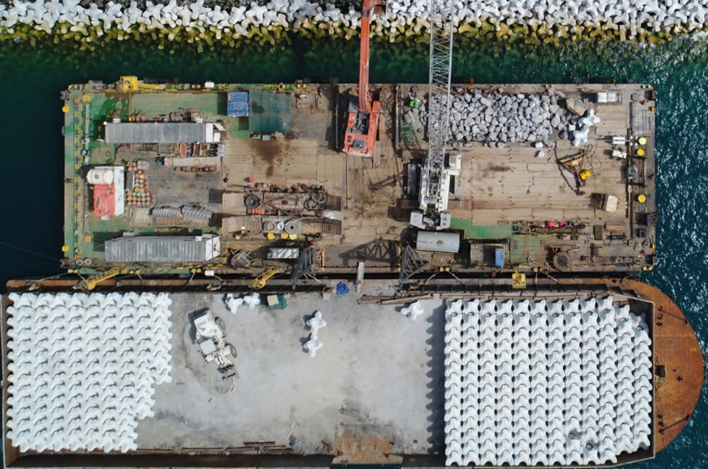
Figure 10: photograph of ACCROPODE™ unit placing using a crane mounted on a barge
